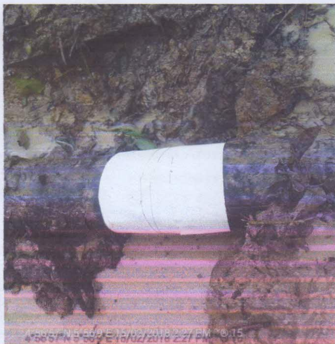
Fig C: Incident facility shortly after repair
